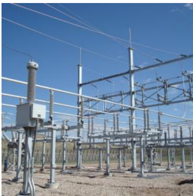
Edison Mission 138 kV Muddy Creek Interconnect Switchstation.
