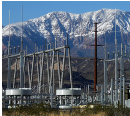
POWER designed the facility and yard for the SVC addition at St. George 138 kV Switchyard.
