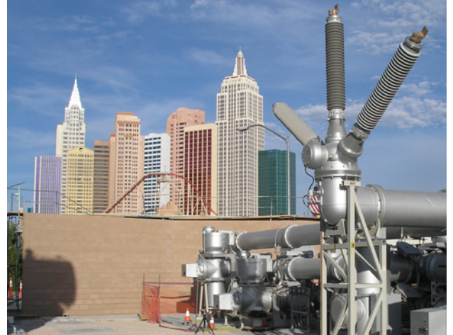
The new Sinatra Substation takes shape on the Las Vegas Strip. Using GIS technology, POWER's design accommodates 500 MVA of transformation in a 1.5-acre footprint.
